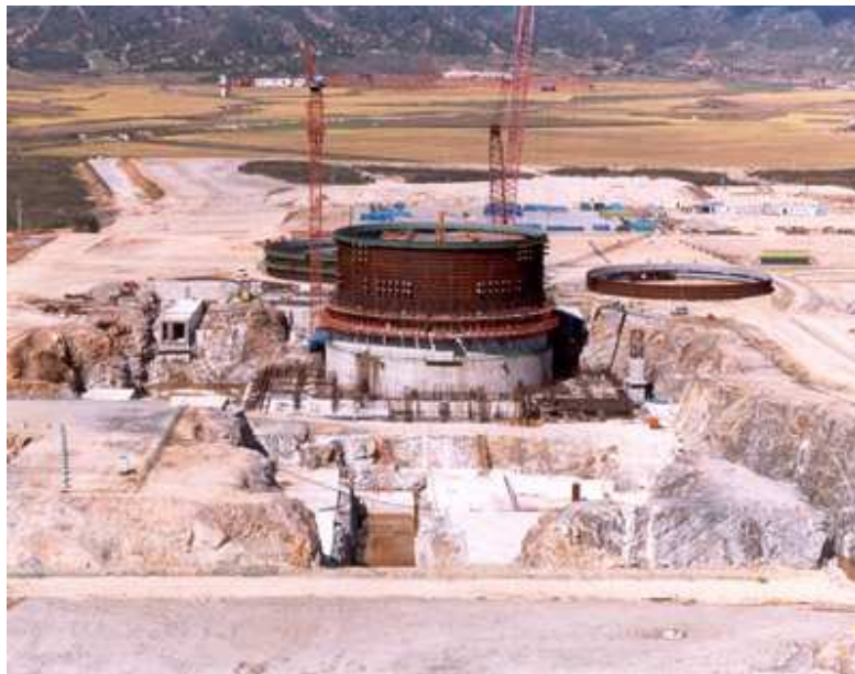
Construction site of the KEDO light water reactor, Kumho Area, North Korea (photo: http://www.kedo.org/lwr_construction_images.asp )
