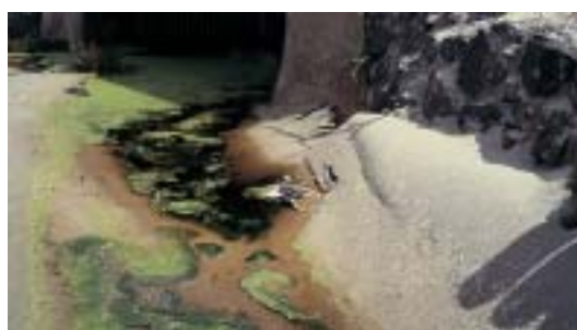
New Plymouth: Old Elliot Street outflow pipe.
