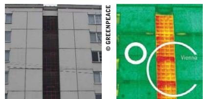
LEFT: THERMOGRAPHIC PHOTO OF VIENNA AM SCHÖPFWERK RESIDENTIAL ESTATE. AS WELL AS LOSSES OF HEAT ENERGY THROUGH THE WINDOWS THERE ARE DIVERSE HEAT BRIDGES IN THE FABRIC OF THE BUILDING.
