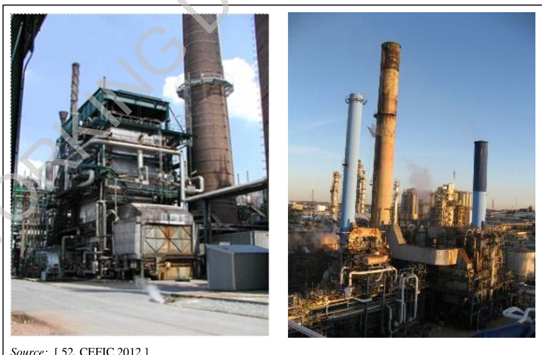
Figure 8.3: Utility boilers in chemical installations
