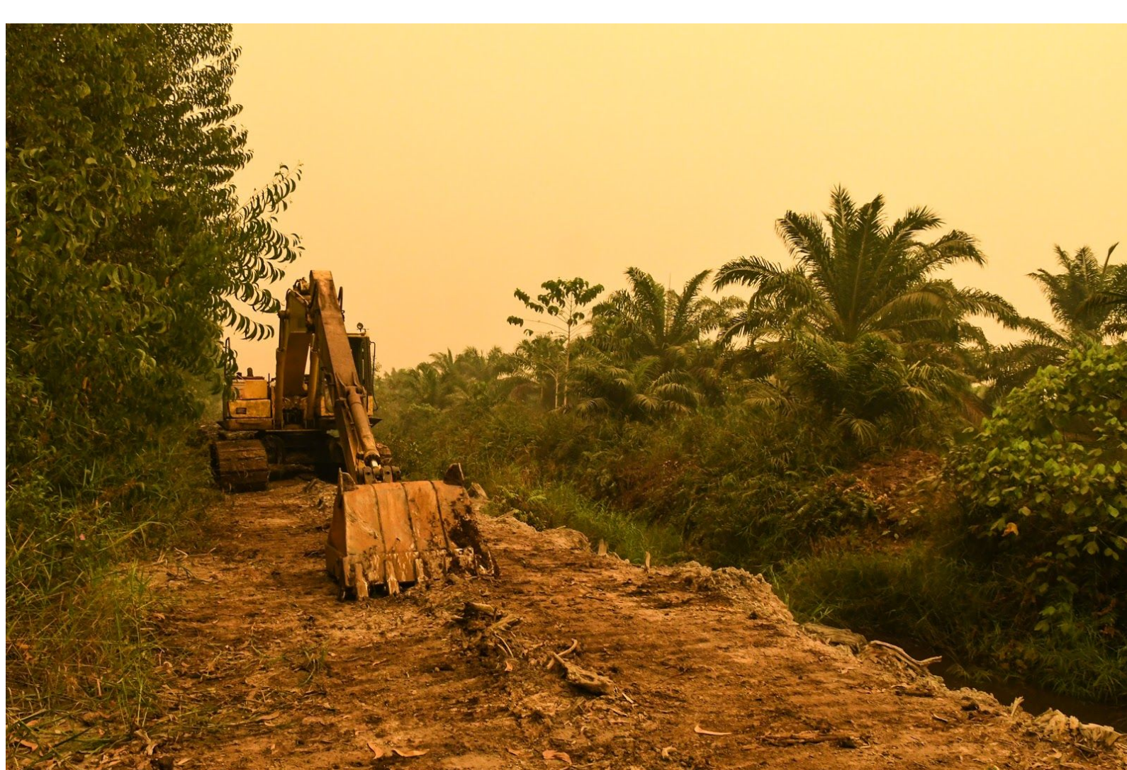
21 September 2019, PT Kaswari Unggul, 1°17'50.699" S 103°45'41.92" E: An excavator at work in the haze from peatland fires in the PT Bukit Barisan Indah Prima concession in Jambi. The plantation company is currently facing civil court action. PT Kaswari Unggul is named as a supplier to Unilever, Mondelēz, Nestlé and Procter & Gamble as well as Wilmar, GAR and Cargill.
