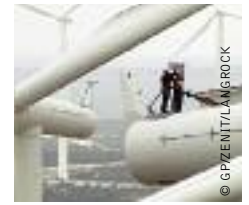
image FOREST CREEK WIND FARM PRODUCING 2.3 MW WITH WIND TURBINES MADE BY SIEMENS. WORKERS WORKING ON TOP OF WIND TURBINE.
