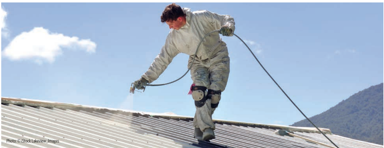
Photo 4. Cool-roof technologies are one alternative strategy cities can use to reduce temperatures. Cool roof coatings can be simply a layer of white paint, as shown here. There are also a variety of shingles and other coverings that are more reflective than traditional building materials.
